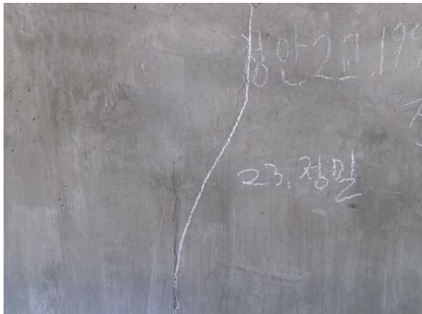
P2 균열 (CW=0.3mm)
