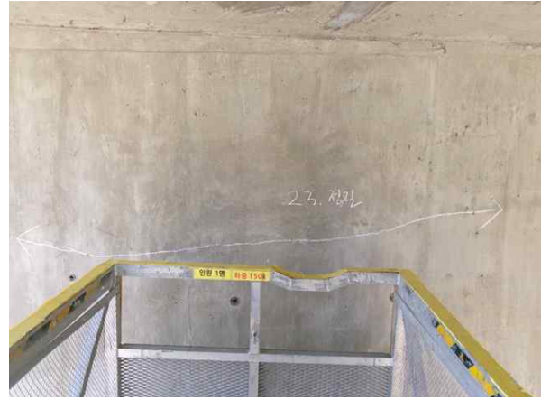
P2 균열 (CW=0.2mm)
